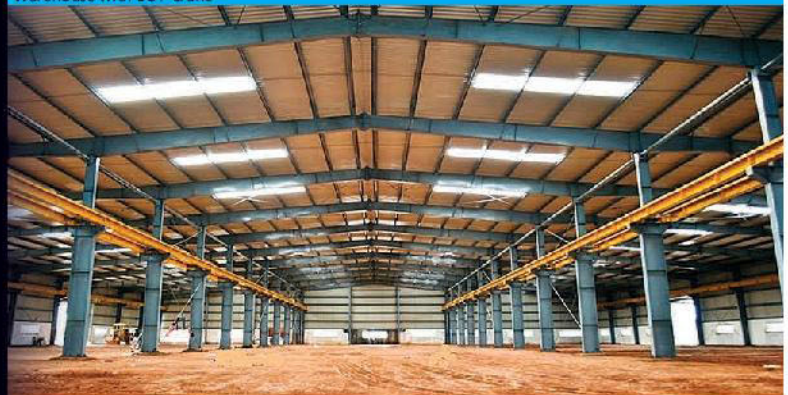
Warehouse with EOT Crane
