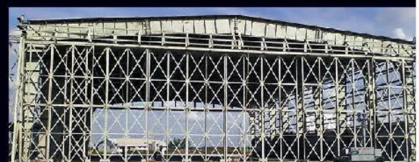
Aircraft hangar with motorised
